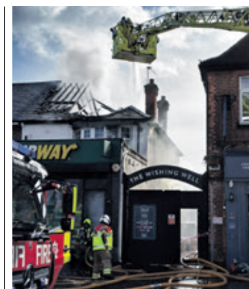
The fire caused significant damage to flats above the Subway shop Credit London Fire Brigade
