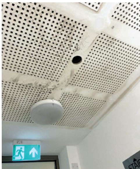
The hole in the ceiling which water poured out of
